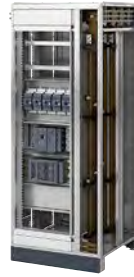
3VA outgoing feeder panels 3NP1 modular installation devices
