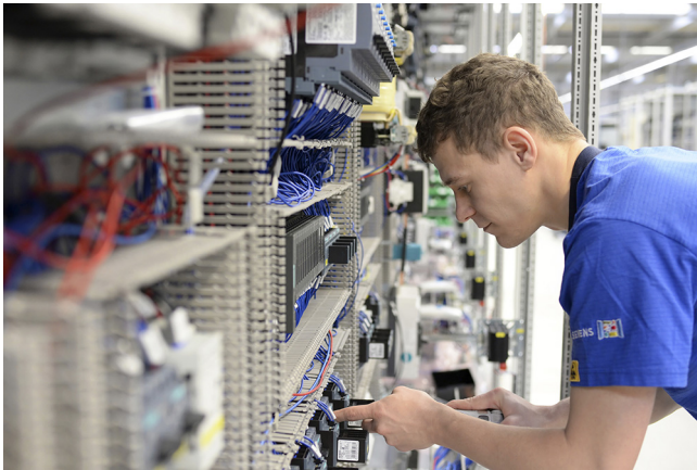
WKC - Control cabinet wiring
