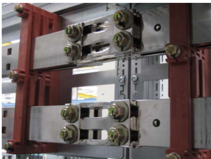
Figure 8-49 M80 - M87, DC busbar
