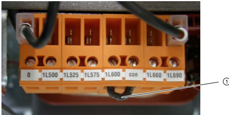
Figure 4-7 Setting terminals for the fan transformers (500 to 690 V 2 AC)
