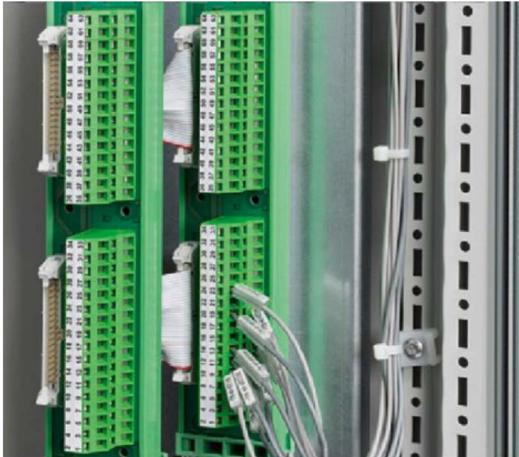
Figure 10-92 Terminal Module Cabinet
