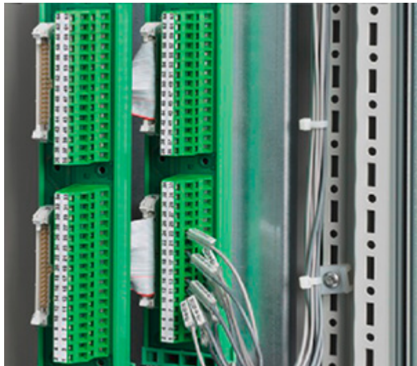
Figure 10-92 Terminal Module Cabinet
