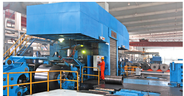
Steel plant motor application
