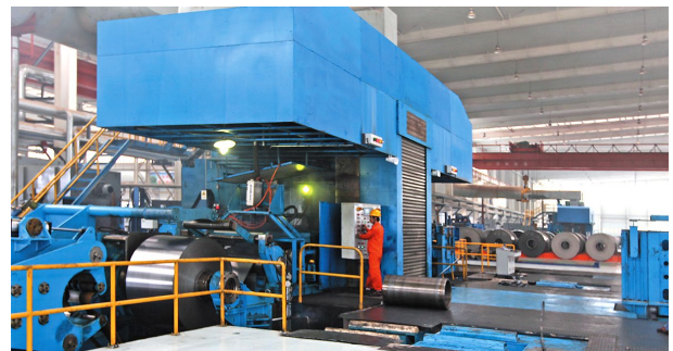
Steel plant motor application
