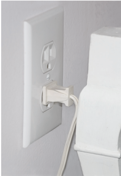
Damaged power supply cord
