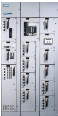
Smart Motor Control Centers Provide Access to Energy Based Information
